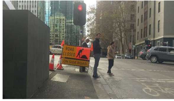
FIGURE 8: EXAMPLE OF TEMPORARY SIGNAGE OBSTRUCTING THE FOOTPATH
