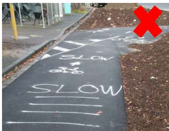
FIGURE 5: INADEQUATE USE OF PAVEMENT MARKINGS
