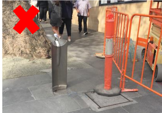
FIGURE 16: FOOTPATH NARROWED THROUGH CONSTRUCTION WORKS WITH NO CLEAR ROUTE FOR PEDESTRIANS
