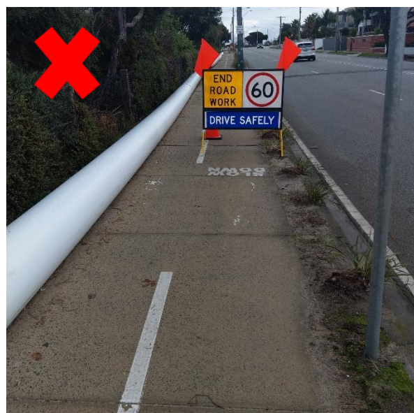
FIGURE 20: TEMPORARY SIGN LEAVING INADEQUATE WIDTH ON SHARED PATH FOR PEDESTRIANS AND CYCLISTS
