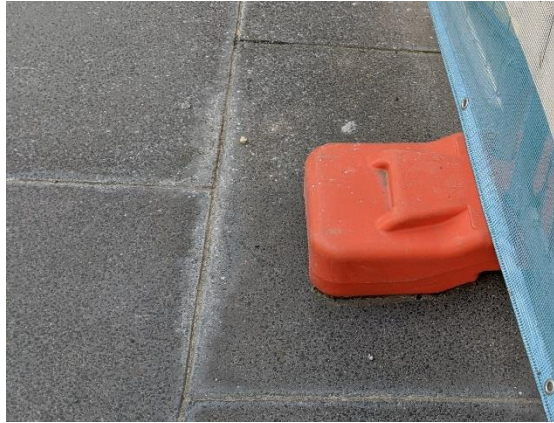
FIGURE 25: FENCE FOOTINGS CAN BE A TRIP HAZARD IN HIGH PEDESTRIAN FLOW AREAS
