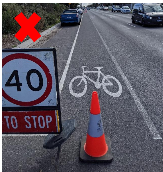
FIGURE 19: TEMPORARY SIGNAGE OBSTRUCTING CYCLE LANE FORCING BIKES INTO VEHICLE LANE
