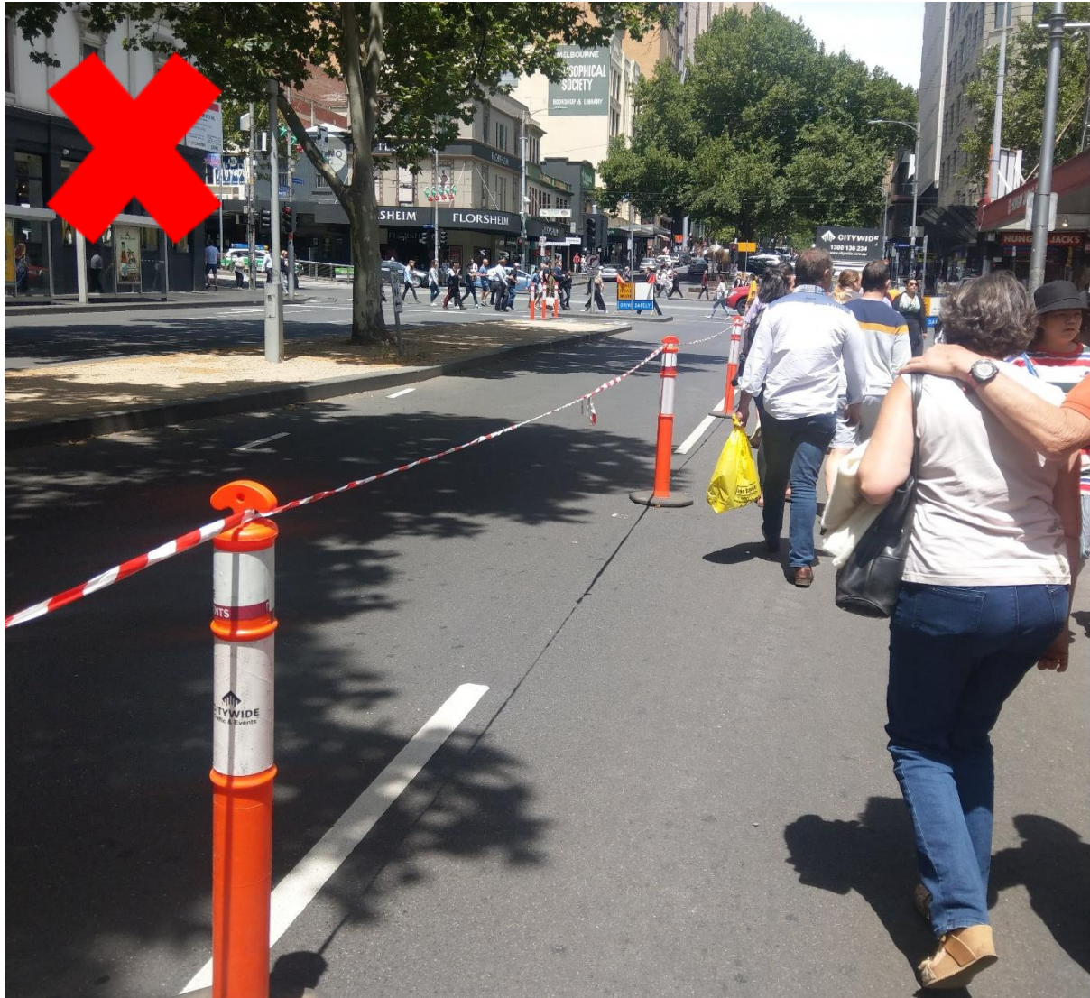
FIGURE 24: INCORRECT USAGE OF TAPE ADJACENT TO LIVE TRAFFIC LANE
