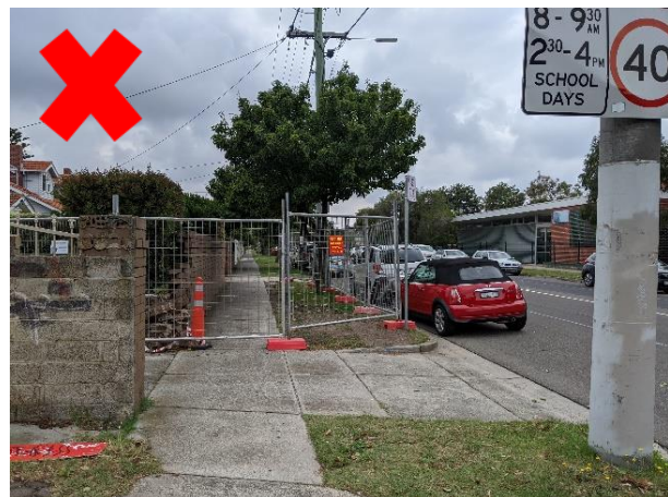
FIGURE 9: NO CLEAR ROUTE EXCEPT IN ROAD - ENSURE CLEAR, LEGIBLE ROUTES FOR PEDESTRIANS IF THE FOOTPATH IS CLOSED
