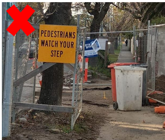
FIGURE 8: OBSTRUCTED ROUTE AND UNEVEN SURFACE - DIVERSION PATHS SHOULD BE SMOOTH AND CLEAR OF OBSTRUCTIONS
