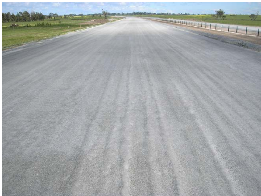
Figure 11 : Excessive Slurring of Fines
