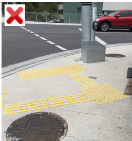
Figure 37: Tactile studs with insufficient luminance contrast to their base surface
