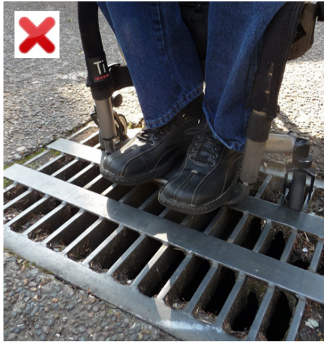
Figure 18: Service grate with size of openings greater than 13 mm
