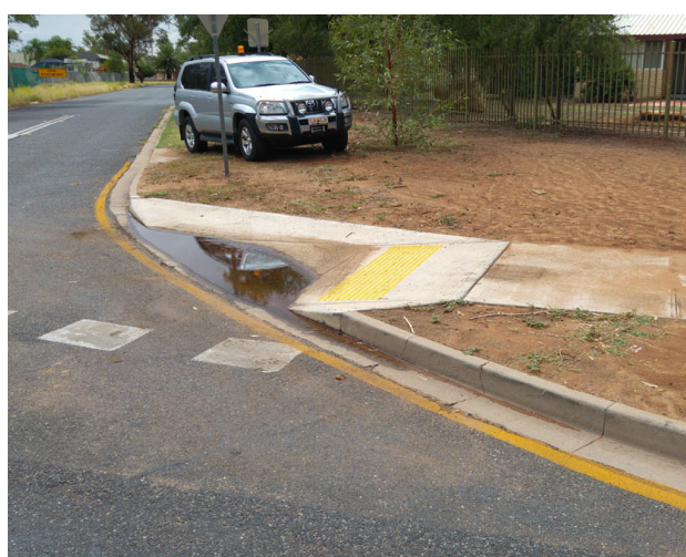
Figure 24: Compliant kerb ramp causing drainage issues
