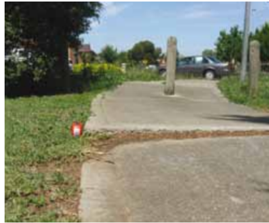
Figure 17: Abutting surfaces not level
